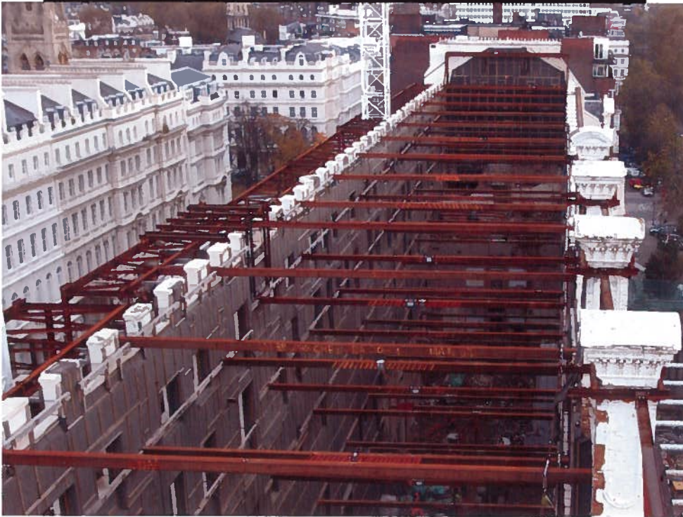
The facades were retained by 500 tonnes of steelwork. Flying buttresses retained the rear wall with horizontal flying shores providing lateral stability
